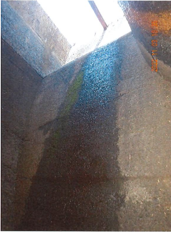
Photo 16 description: Left Side Interior Left Riser Box
