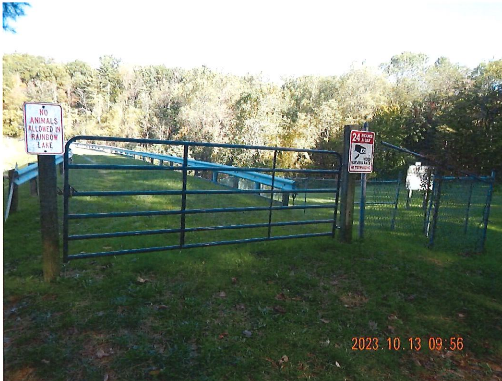
Photo 39 description: Warning Signs and Locked Gate at Access to the Dam Crest
