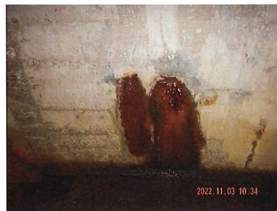
Photo 24 description: Seepage Point Left Side Interior Left Box Spillway
