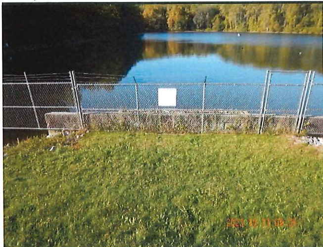
Photo 40 description: Warning Sign on Safety Fence at Principal Spillway
