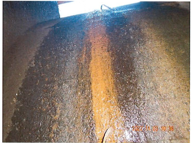
Photo 19 description: Back Side Interior Left Riser Box
